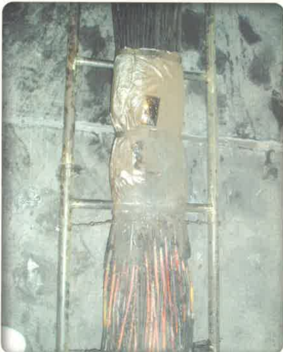
▲ Back side section after Fire Test
