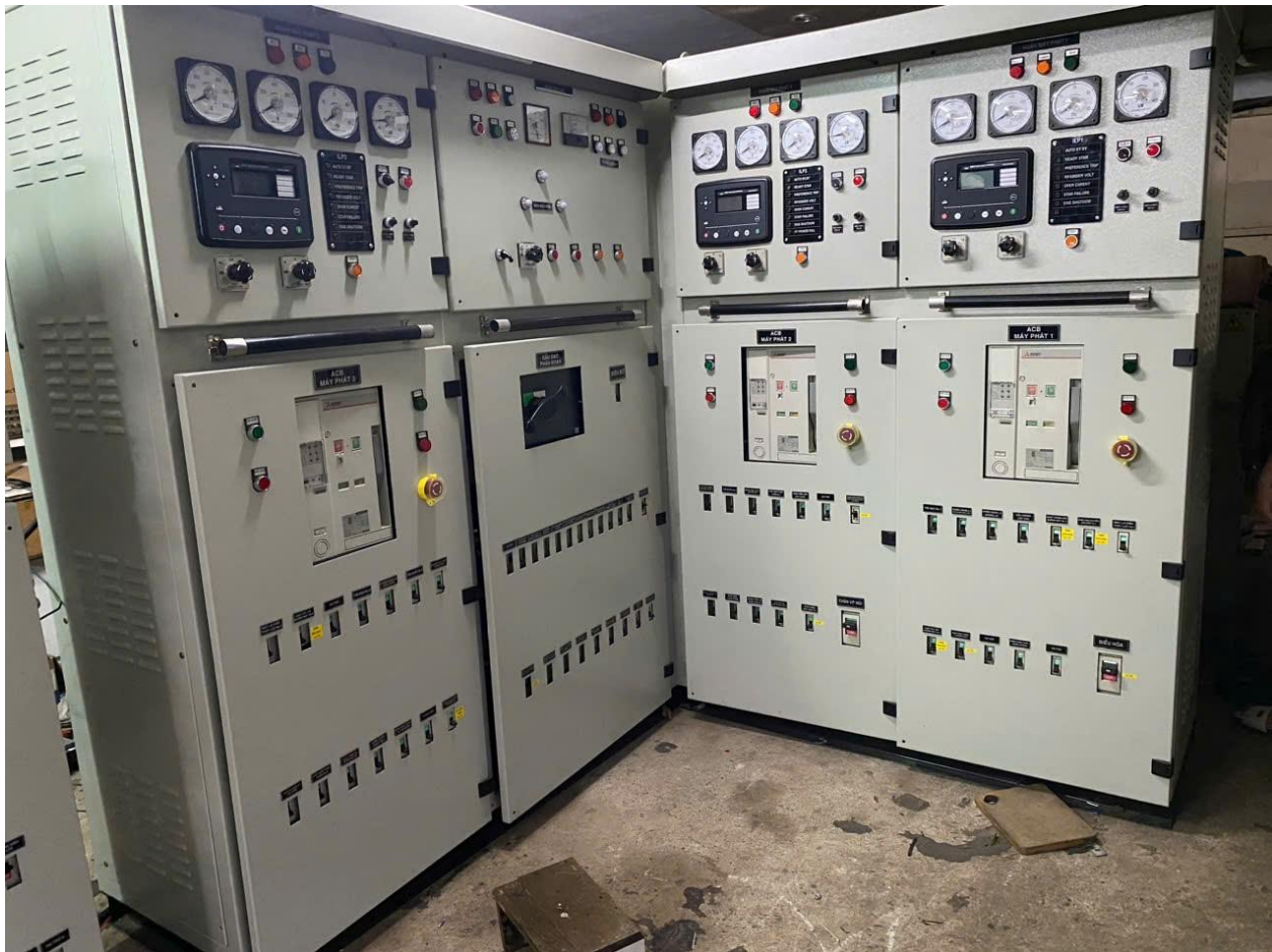
Main electrical cabinet of Viking Tonle
